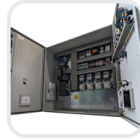
Photovoltaic Panel System G99 - Coupling Panel
